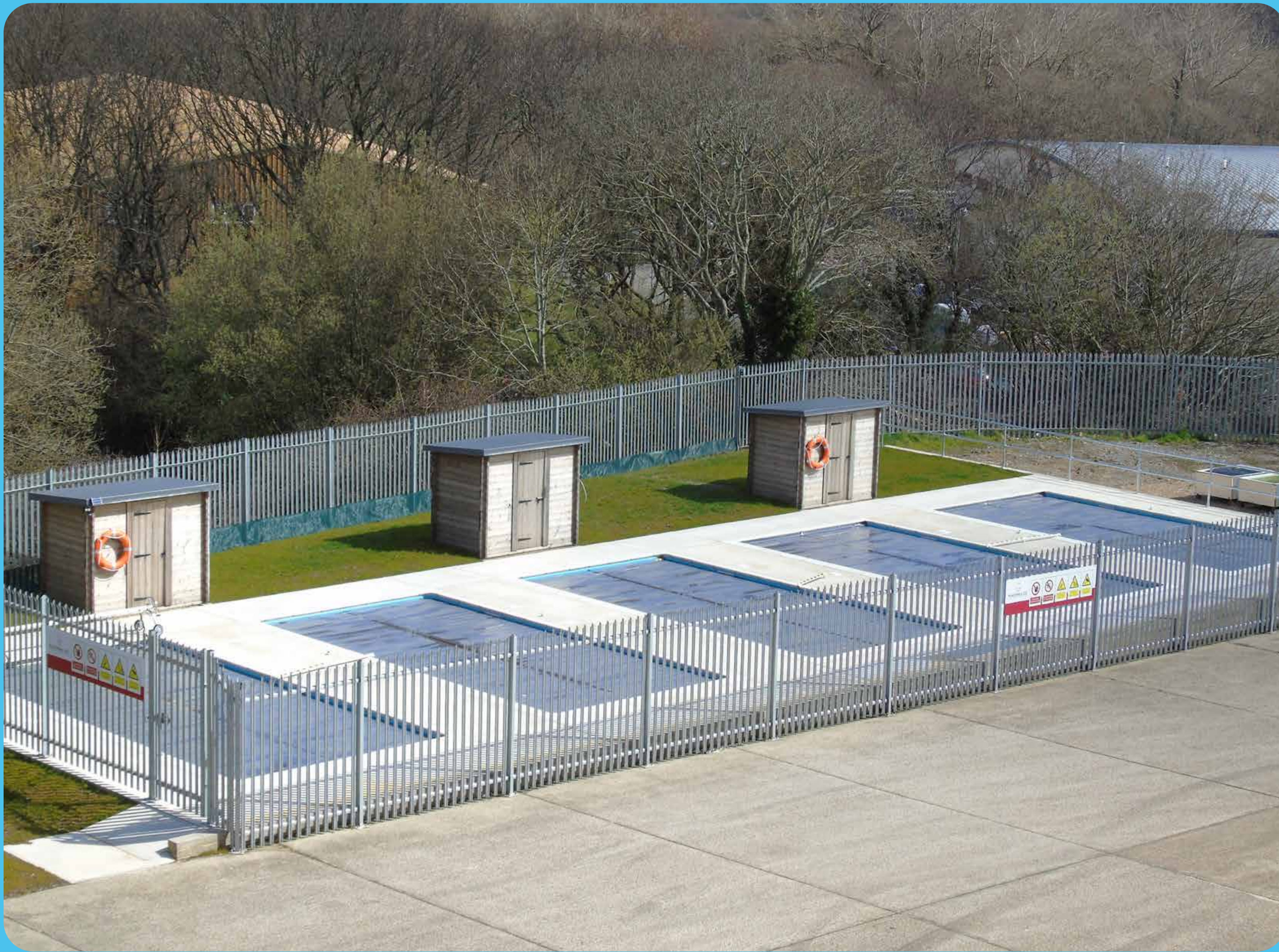
Figure 3. Bespoke testing facility, Plastipack Ltd, Hastings UK.
